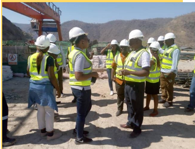
Delegates from Malawi appreciating one of the electricity generation flagship programs being implemented at Kafue Lower Gorge in Zambia
